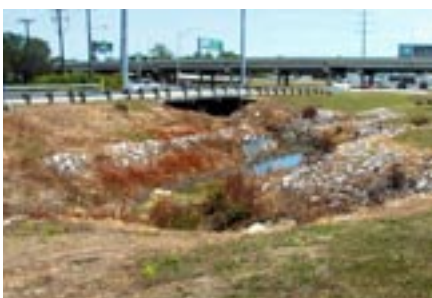
This stone-filled open ditch at Rivers Avenue near the headwaters of Filbin Creek could be augmented with detention areas, vegetated swales, and live oaks along the banks.
