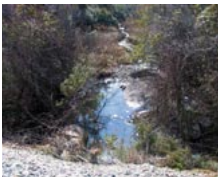
Stormwater outfall pipes at edge of marsh are laden with sediments, resulting from accelerated runoff rates.
