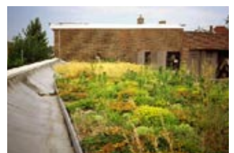
Image of a green roof installation
