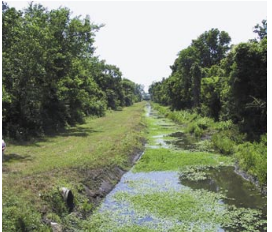
Image shows a channelized section of Filbin Creek, choked with aquatic weeds. Stormwater quality elements, including wetlands and native vegetated open areas could reduce the nutrient loading which contribute to the excessive weed growth.
