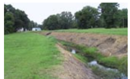
This channelized section of Filbin Creek was purposely incised and disconnected from its floodplain to enhance stormwater conveyance. Our understanding of stream functions have since changed. The result of channelizing channels around the world is an unstable stream with eroded slopes and increased downstream sediment loads. Establishment of natural stream geometry and re-connection to the floodplain would help to restore this ditch to a healthy stream system.
