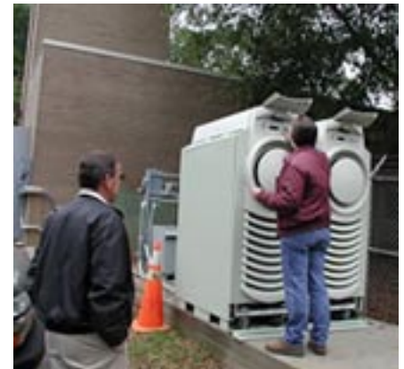
Two 28kW microturbines provide power for a fire station in Charlotte, NC
