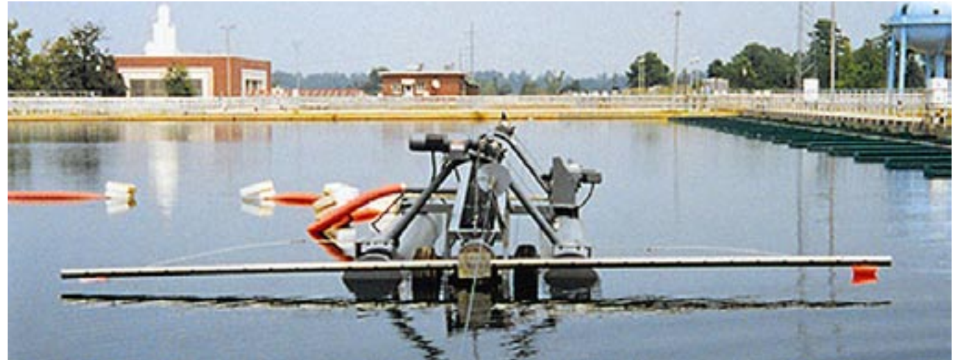
The Hanahan Water Treatment Plant's FLUMPs remove solids from the water supply
