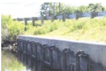
Flap gates near mouth of Filbin Creek prevents tidal flow upstream. While the flap gates may prevent upstream tidal flooding, they also eliminate estuarine intertidal wetlands – an alternative that allows active operation of the flap gates could potentially provide both functions.
